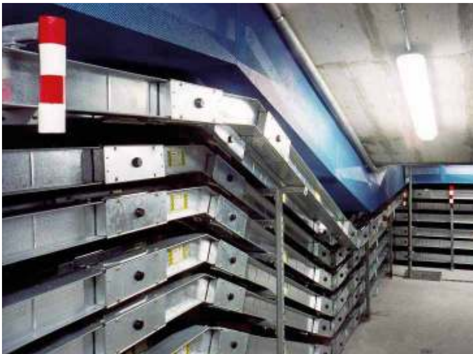
Example of high power distribution
